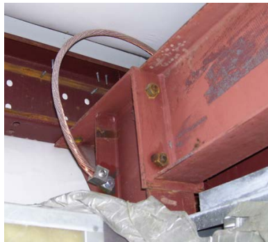
Bonding jumper installed between buildings
