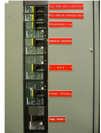
Identification and labeling of circuits
