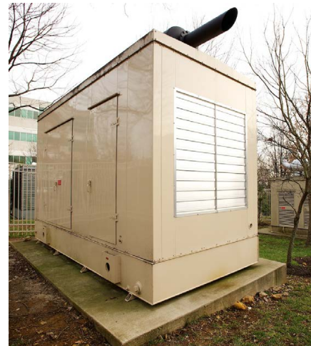
New emergency generator
