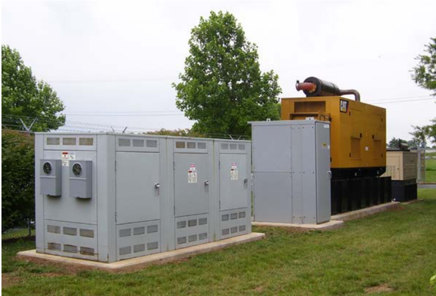
NOC's outside emergency generator
