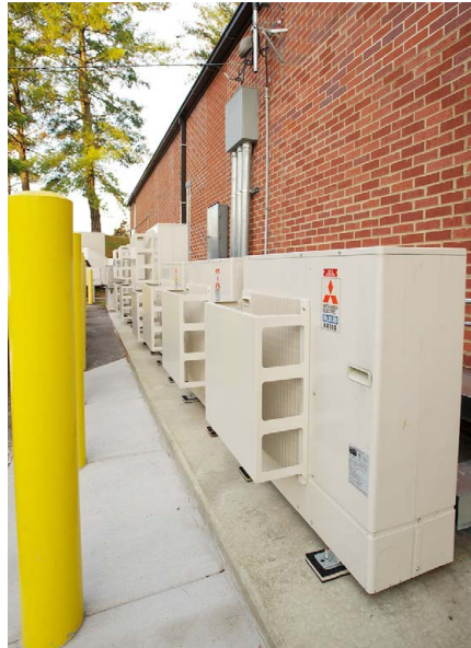
Mitsubishi exterior units
